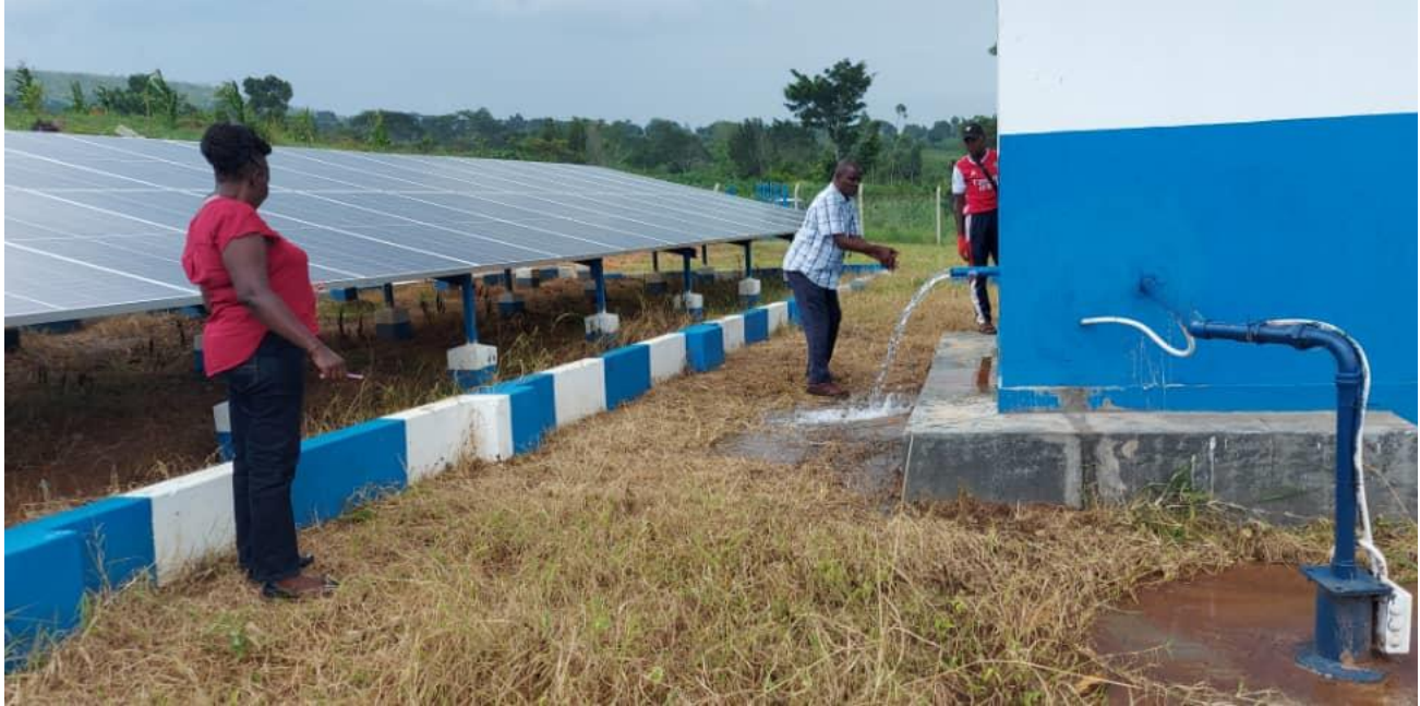
Matongo water supply system to serve eight villages of the parish
